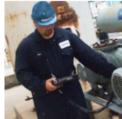
Rotating Equipment Inspection
